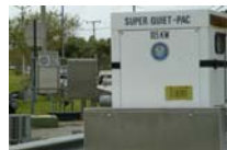
Generator powers a sewer lift station, Florida Courtesy FEMA
