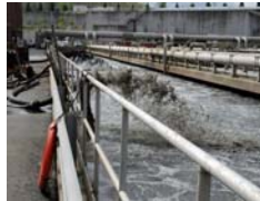
Flooded treatment plant, Atlanta Courtesy FEMA
