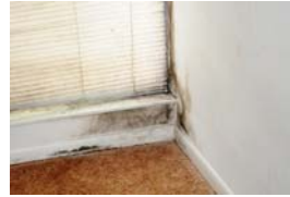
Visible mold after flood, Tennessee Courtesy FEMA
