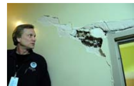
Earthquake damage, California
