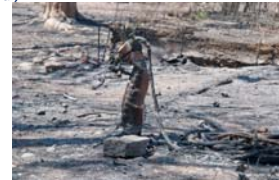
Fire damaged well water pump at child care center, Texas Courtesy FEMA
