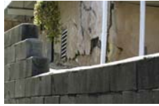
Foundation damage after landslide, California Courtesy FEMA
