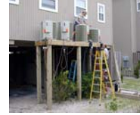
HVAC protection, North Carolina
