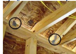
Hurricane clips, Florida
