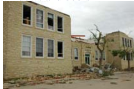
Damaged windows at an elementary school, Kansas Courtesy FEMA
